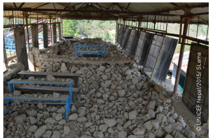
School building destroyed by 2015 earthquake in Sindhupalchowk.
